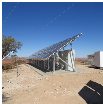
Hybrid Solar Power System, Cradock SA
