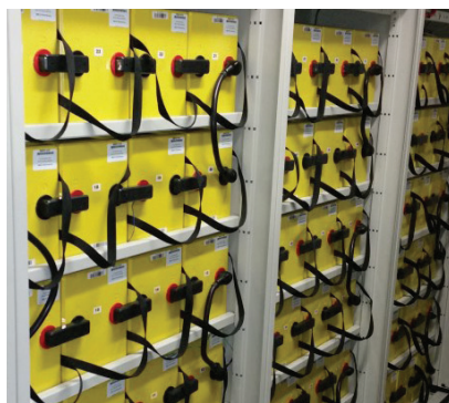
New batteries installed
