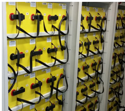
New batteries installed
