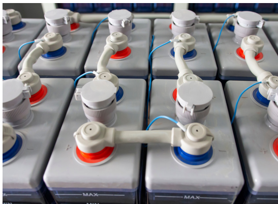
New DC power plant
