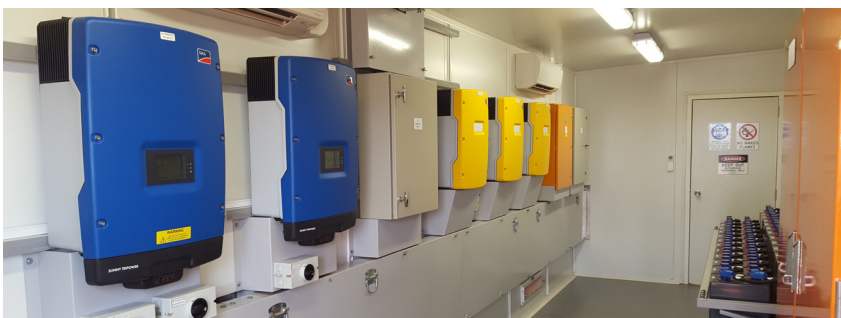
Fully-transportable solar-powered retail fuel outlet at Onslow, Western Australia.
