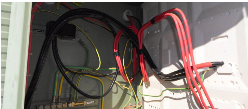
Mobile Communications Facility - Bergalia NSW
